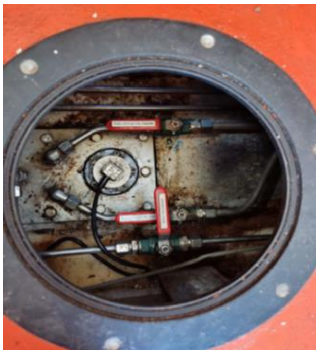
Daughter craft fuel isolation valves showing in the open position.
